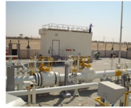
Supply of Gas to New Al Ain Cement Plant for Arkan
