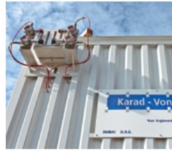
Shell Majnoon Facilities Packaged Substations
