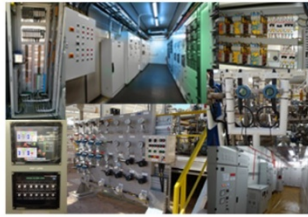
Automation, Instrumentation and Control System Projects
